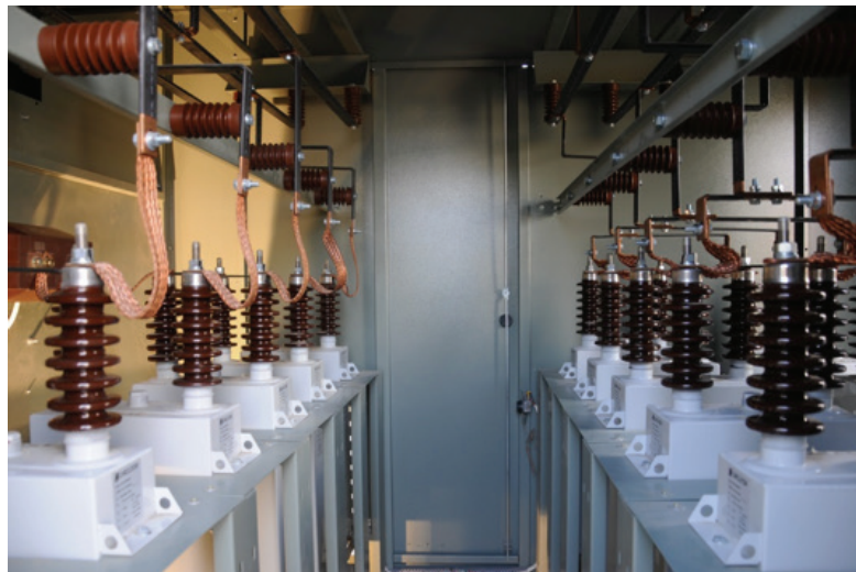
Fig. 4 Compensating capacitors perform power factor compensation at a utility switching yard.
